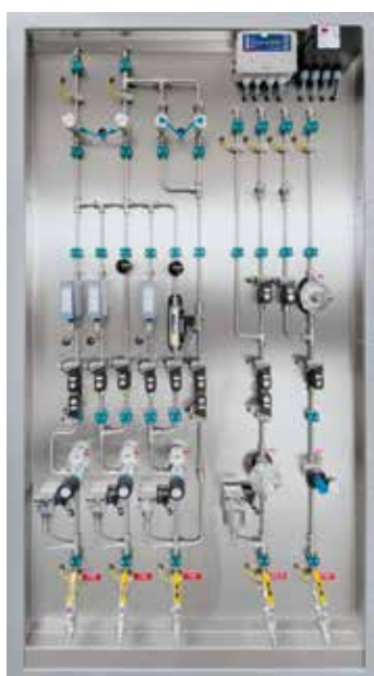
Gas management system
